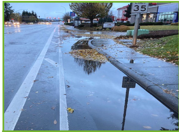
Leaf accumulation causing flooding
