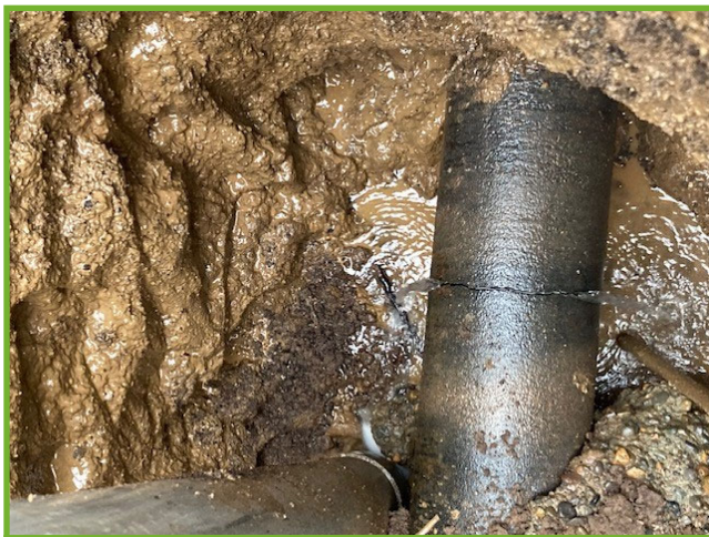
Crown break in main
