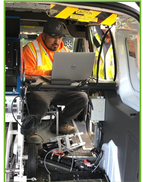
Operating the CCTV system
