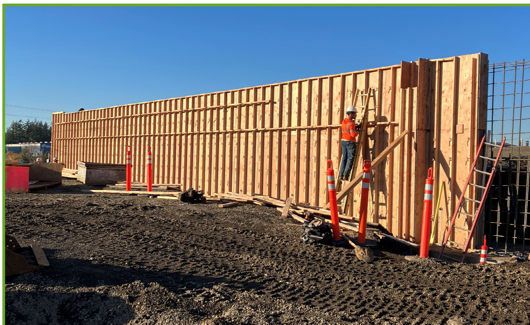
Form of the retaining wall between the public parking area on the upper level and the work yard on the lower level.
