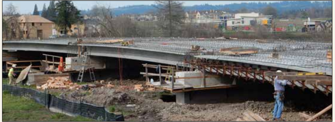
The Barber Street bridge and road extension project near Villebois is on schedule to open this fall.
