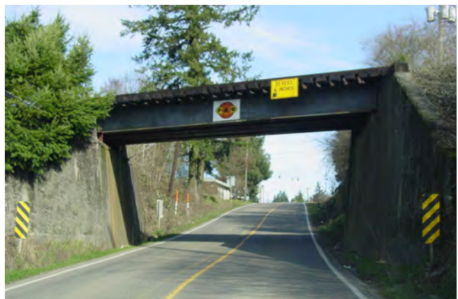
The railroad bridge over Grahams Ferry Road has limited horizontal and vertical clearance. This creates a safety hazard, particularly for bicyclists, pedestrians, and freight traffic.
