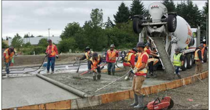
Construction workers pouring and preparing concrete at the new Boeckman Road roundabout at the northern end of the Kinsman Road extension project.
