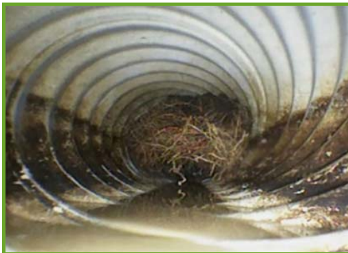
Before— roots obstructing flow
