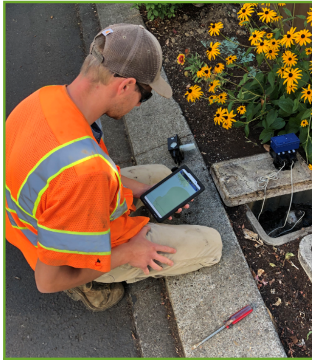
AMI radio installation
