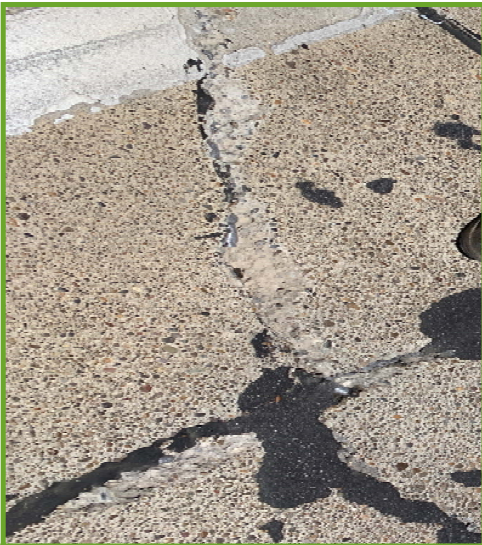
Crack in need of repair on 95th Ave
