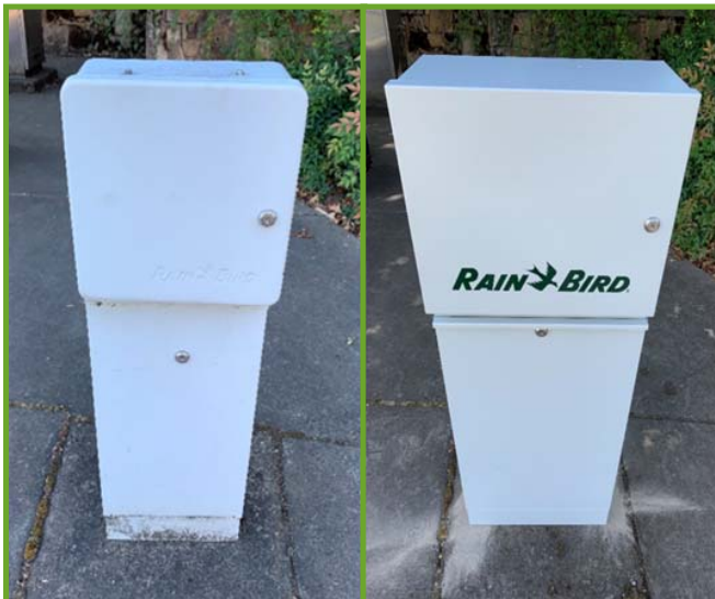
Irrigation Controller Upgrade
